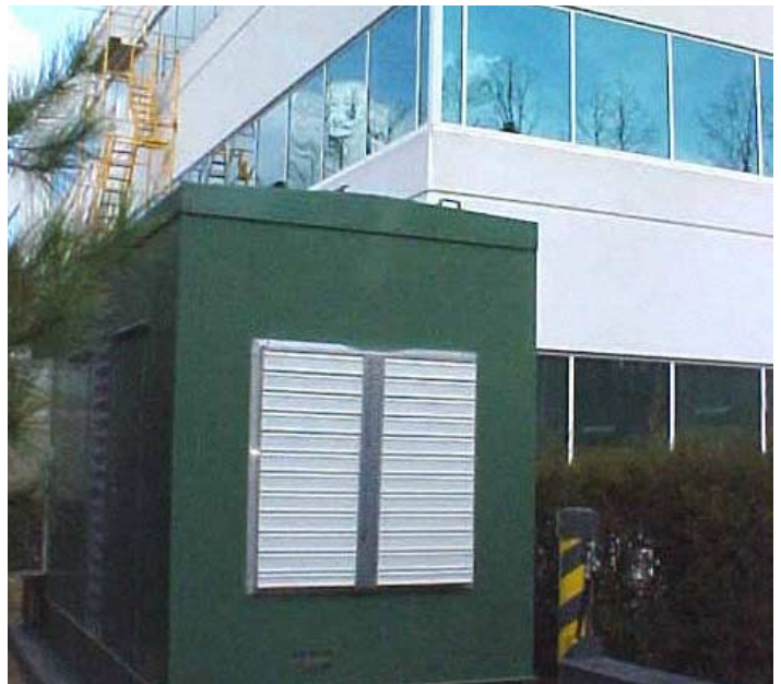
The Cat solutions package is a self contained unit that sits outside the facility.
